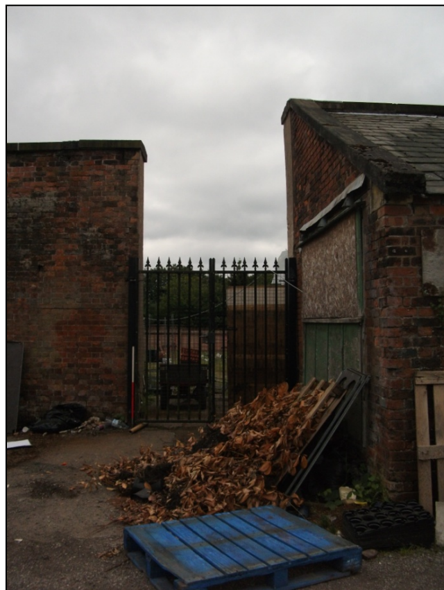
Fig 14: Blocked doorway on Eastern Elevation of the Potting Sheds, looking S.
