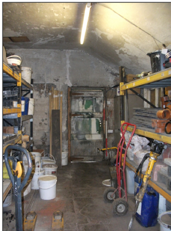
Fig 43: Interior view of the Potting Shed along the gardens Northern Elevation, looking W.
