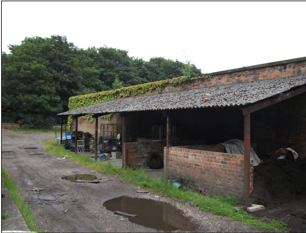
Fig 15: Lean to Shed at eastern end of the gardens North Elevation, looking SE.
