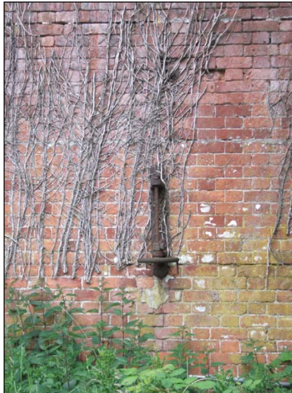
Fig 38: View of ventilation apparatus along the southern face of the gardens central wall, looking N.
