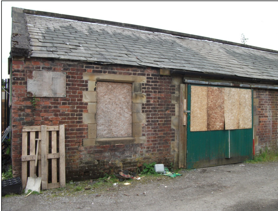
Fig 13: Sliding double door at eastern end of the Potting Sheds North Elevation, looking SW.
