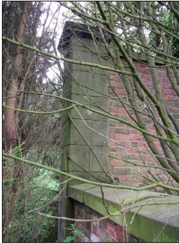
Fig 25: View of sandstone pilaster at southern end of the gardens Western Elevation, looking W
