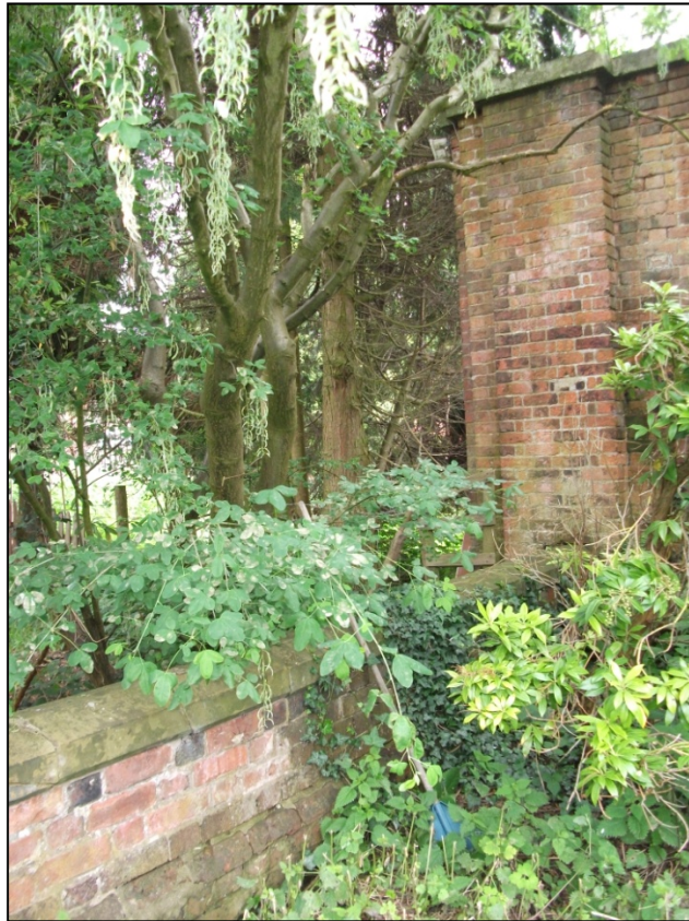
Fig 27: View of break in gardens Western Elevation, to the rear of the Garden Cottage, looking NE.
