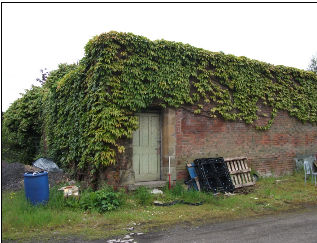
Fig 16: Later inserted doorway at eastern end of the gardens Northern Elevation, looking SW.
