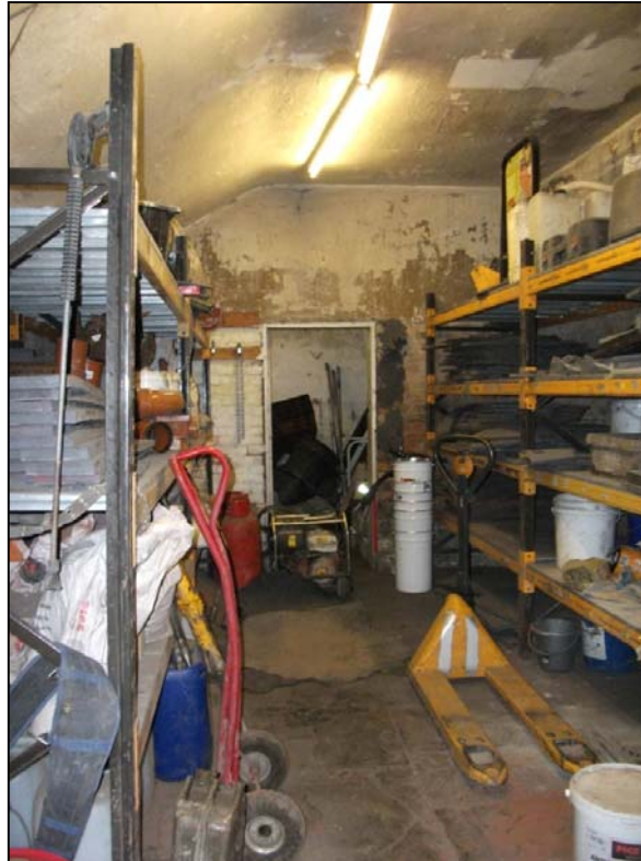
Fig 42: Interior view of the Potting Shed along the gardens Northern Elevation, looking E.
