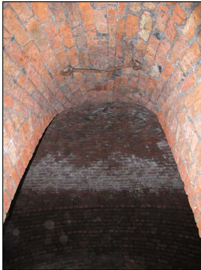
Fig. 17 – Shot of approach chamber barrel vaulted roof and iron bar fixture. Looking south.
